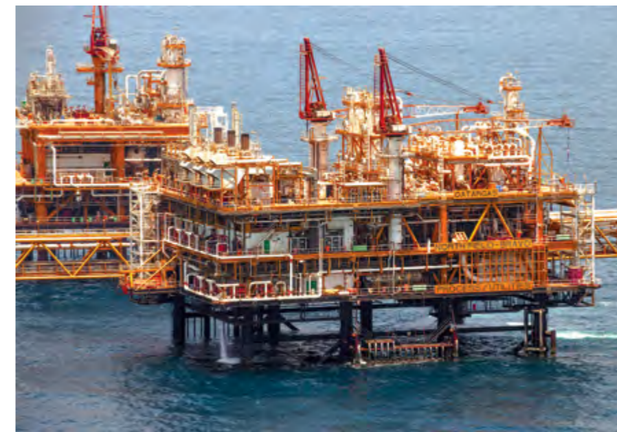
Wellheads and christmas trees can be seen on a Qatargas offshore facility.
