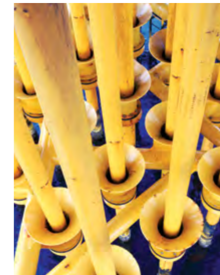
A gas well is a series of concentric pipelines, which reach from ground surface to the gas producing formation.
